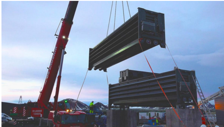
< Construction is underway for Climeworks’ new direct air capture and storage plant in Iceland called Orca . Shopify has made a multi-year commitment to purchase 5,000 tonnes of carbon removal from Climeworks to help Climeworks continue to scale their gold-standard solution.
