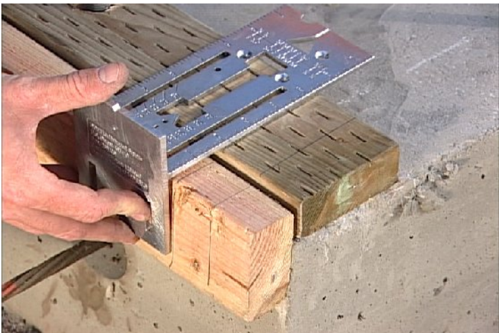
With sole plate in place over foundation bolt, tack top plate on the side of slab with nails.
