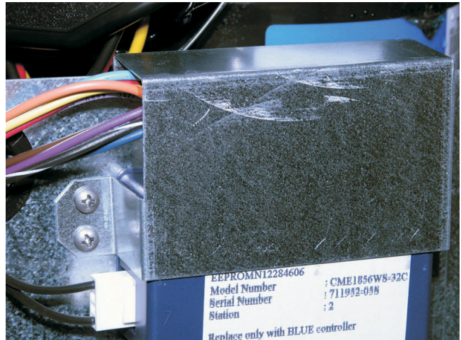
Cover Installed on Unit
