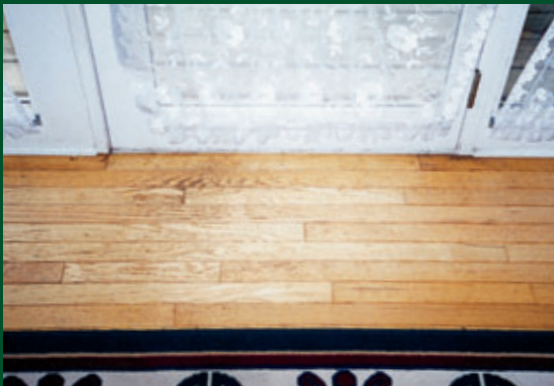
Dirty floors with finish totally worn off.
