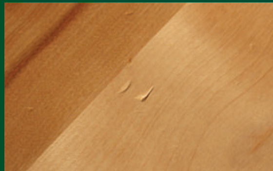
Dents (these usually require board replacement).
