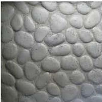
Grout is recessed
