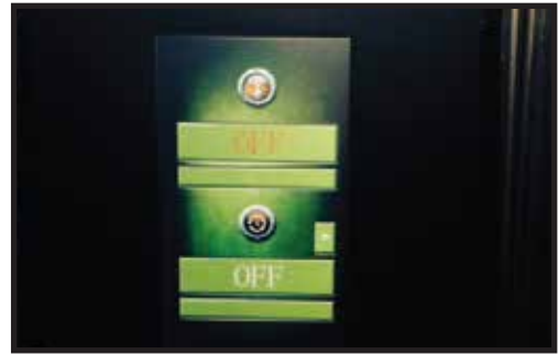
Digital Control Panel
