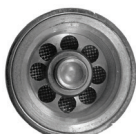
clear valve no blockage
