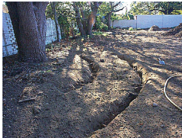
Trenches are being located around this existing tree to accommodate an electrical conduit.
