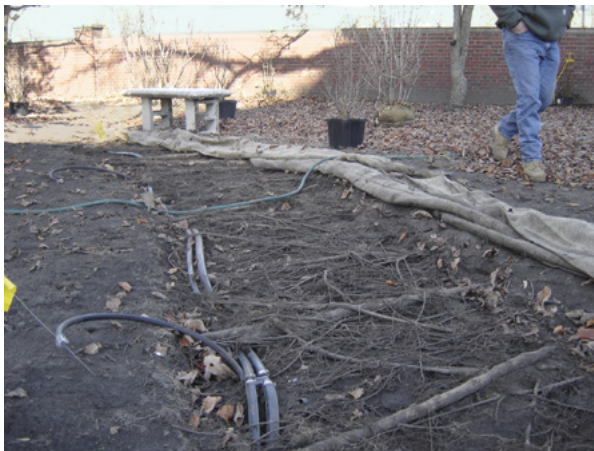
At the Radcliffe Institute, the foundation for a new path was excavated using an AirSpade. Irrigation lines were snaked through the exposed roots, and minimal root pruning was completed before installing a gravel root barrier and the top course of stone dust pavement. (Image courtesy of SSA.)
