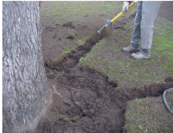
Radial trenching with an AirSpade encourages root growth by breaking through compacted and highly stratified soil layers.
