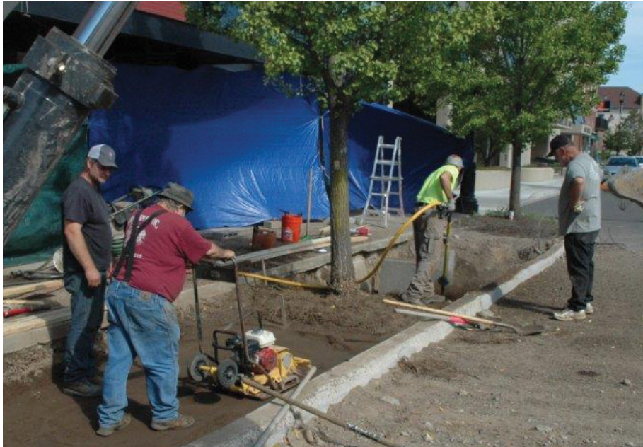
Installation of a new paving system for ginkgo street trees. At the right of the photo, an arborist excavates highly compacted sandy loam soil that had supported brick pavement for over 20 years. At left, the contractor finishes installation of an engineered sand based structural soil, which is to bear the load of new pavement.
