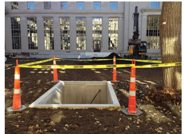
To install this area-way at M.I.T. required diligent tree protection, and intensive excavation using an AirSpade and root pruning by a trained arborist. (Image courtesy of SSA.)
