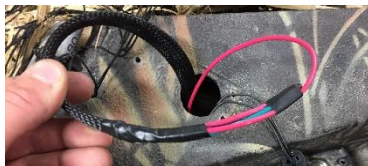
Use a guide wire to lead trim wires though route. (Excel Boats) have a tube with the navigation wires running in them. Use the same route.
