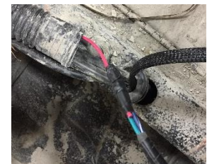
(Excel Boats) Run guide wire through wire housing and pull through trim switch wiring.
