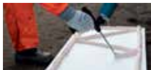
Extrude Soudabond Easy onto the panels and leave to set for ca 5 minutes
