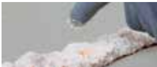
Adhesive layer bursts when touched → too soon
