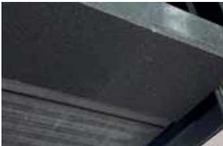
The panel is now firmly installed – while Soudabond Easy continues to cure the Fix All High Grip adhesives keeps the panel in place
