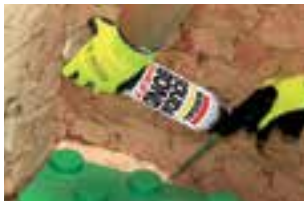
Seal at the side of the panels with Soudabond Easy to create a completely insulated layer
