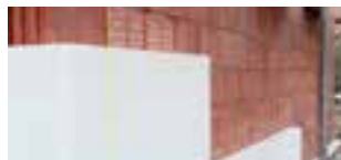
Ca 60 minutes after installation of the panels it is possible to continue working on the wall
