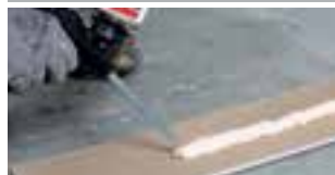
6. Set end screw of the gun to the required extrusion rate (ca 30mm bead) and extrude adhesive
