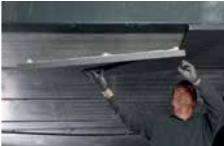
Install the insulation panel ca 5 minutes after the application of Soudabond Easy
