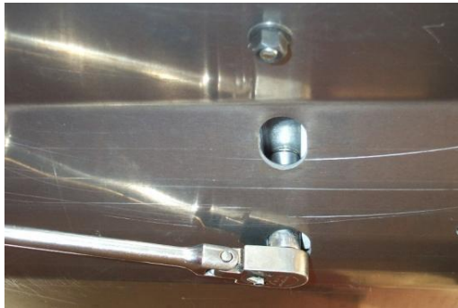
Figure 35 - Two Oblong Holes in the Skid Plate
