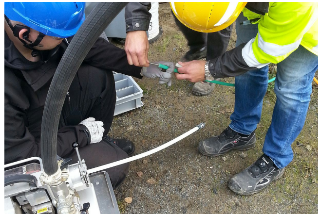
Inserting a sonde into a micro duct before connecting duct to a jetting machine.
