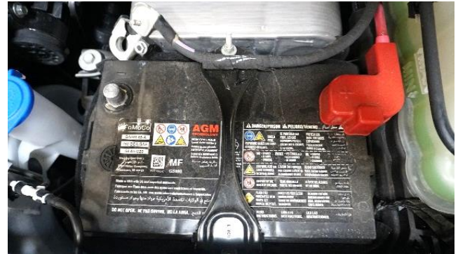
Secondary Battery - Driver Side
