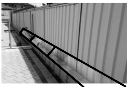
Oscillot® installation with rigid polycarbonate blocking off ledge on raised retaining wall eliminating it as a potential platform.
