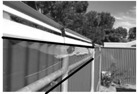
Clear polycarbonate sheeting installed just below Oscillot® eliminating the horizontal rail as a potential 'ladder'.
