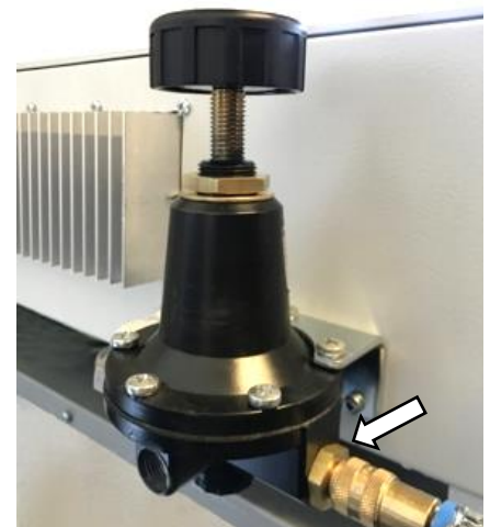
Figure 12: Compressed air connection on the pressure regulator
