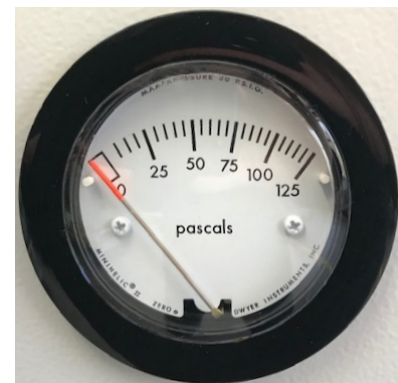
Figure 23: analog pressure display (manometer) for compressed air sweeping on the chamber front
