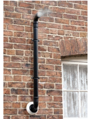
Installed to prevent nuisance pluming across the window
