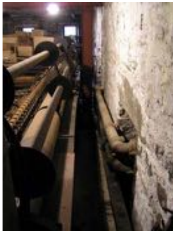
Heating pipes to the rear of the mule served by the boiler in the weaving shed through the original fireplace on the gable
