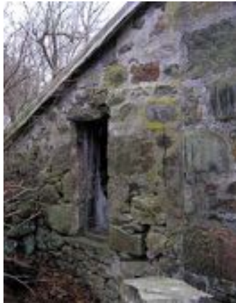
Junction of masonry between the wash house and the main mill structure
