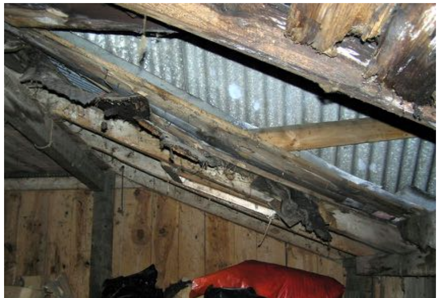
The precarious nature of the attic roof construction, showing clearly the remnants of the original asphaltic roof covering
