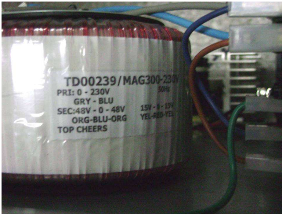
Mains Transformer in Amplifier Module
