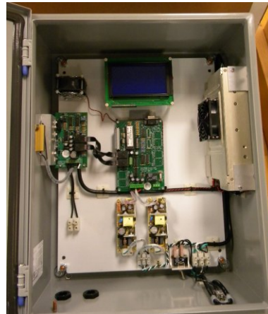
Control unit door open showing electronics inside
