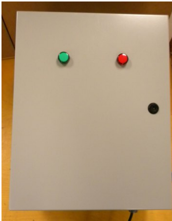
Control unit with door closed
