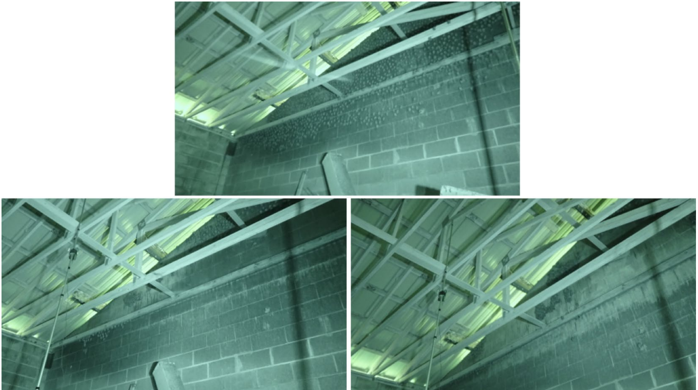
Figure 3-5: Bats roosting at 09:00 on east wall at north end of roost post-treatment. From top, left to right: October 9 (no treatment), October 23 and October 26 (post-treatment).
