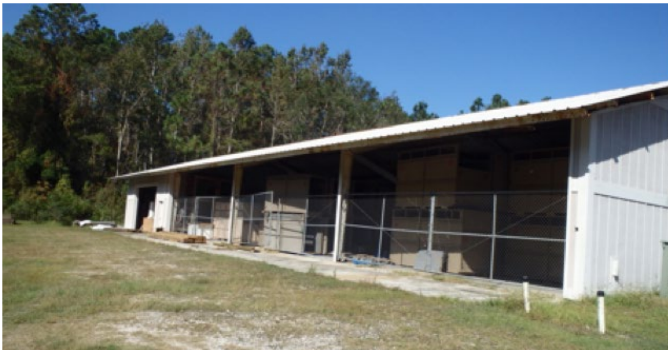
Photo E-1 Maintenance building and crate storage; Garage (far end) used for storage and was location of roosting bats
