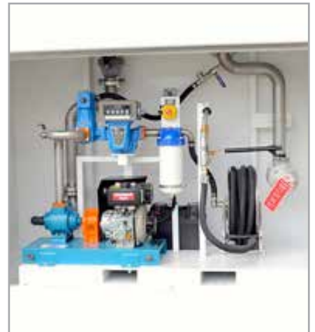
Bunded Pump Bay Housing
