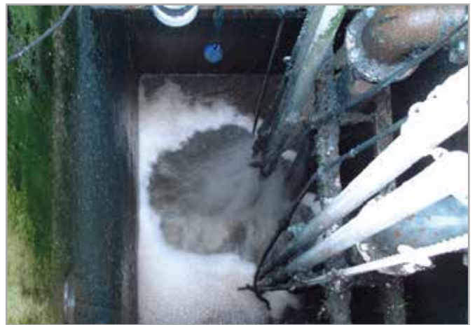
4m wet well pump control and high fill rate
