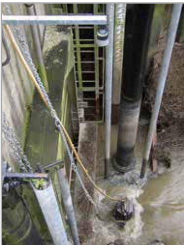
7m Pump Control
