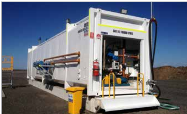
PT Series Integrated Pump Bay
