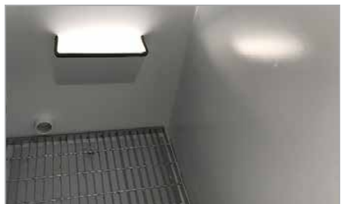
PETRO Store Bunded Pump Bay Housing with Letterbox Style Hose Outlet / galvanised grated bunded floor
