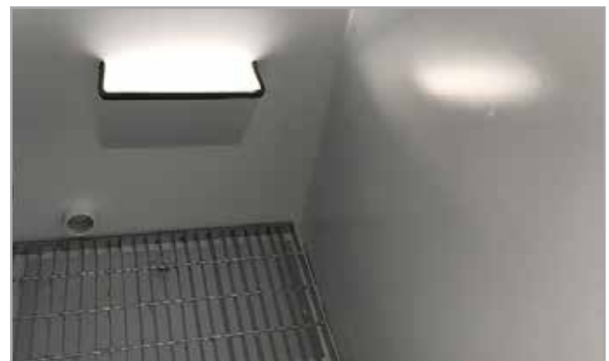
PETRO Store Bunded Pump Bay Housing with Letterbox Style Hose Outlet / galvanised grated bunded floor
