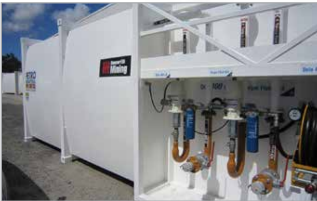
Bunded Pump Bay with Platform
