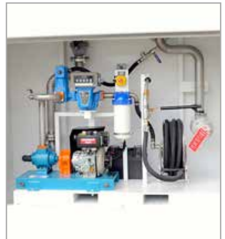
Bunded Pump Bay Housing
