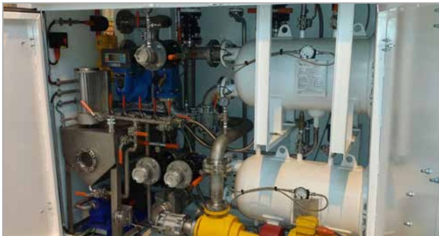
Example of a PETRO Aviation Fuel Sampling, Filtration and Dispensing Module
