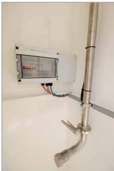
Suction line & electrical junction box
