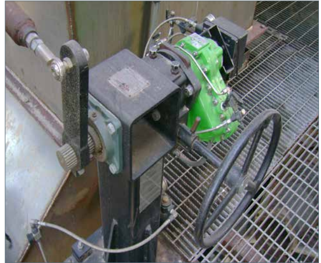
TYPE K PM Series on Primary Air Fan Inlet Damper
