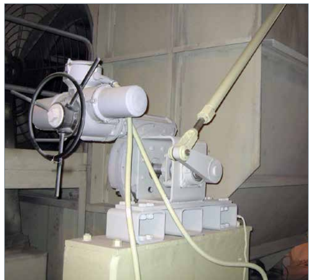
IQ Series on ID Fan Inlet Damper
