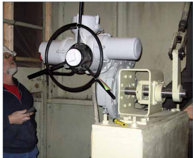
IQ Series on FD Fan Inlet Damper
