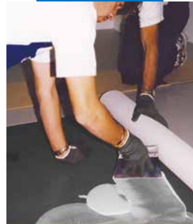
Laying rubber floor covering on Mapelay sheets using Adesilex G19. Note: the joints between the sheets of rubber floorings are staggered with respect to the joints in the sheets of Mapelay
