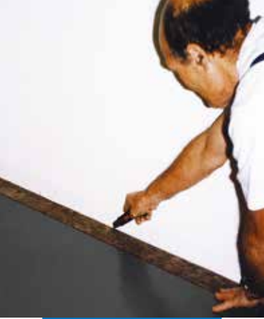
Laying Mapelay and formation of a 5-10 mm joint in correspondence with the constraints of the floor
