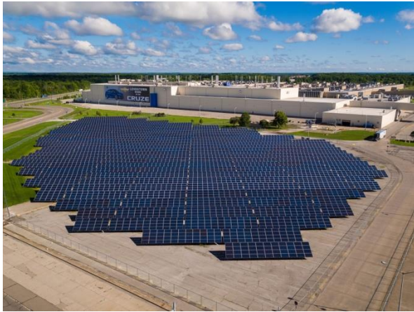
2.2 MW Solar Field General Motors Lordstown Assembly Design / Build / Transfer
