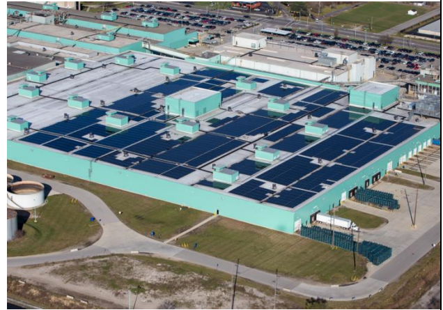
1.7 MW Rooftop Solar Array General Motors Powertrain, Toledo, Ohio Power Purchase Agreement
