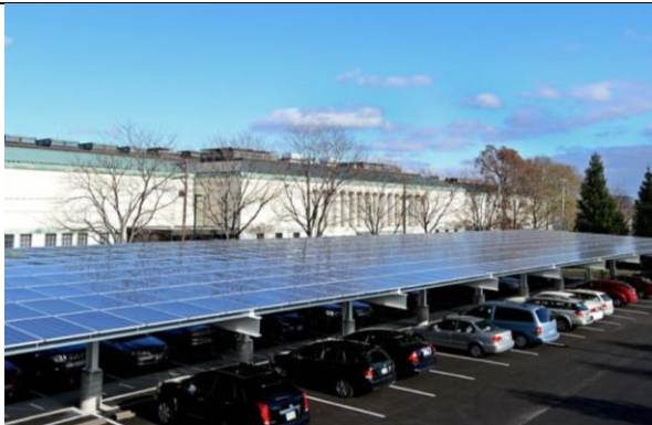
303 kW Solar Canopy Toledo Museum of Art, Toledo, Ohio Power Purchase Agreement
