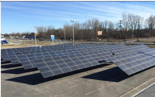
146 kW Ground Mount Solar Array GM Flint Engine Plant, Flint, Michigan Design / Build / Transfer
