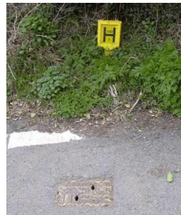
Example of underground fire hydrant
