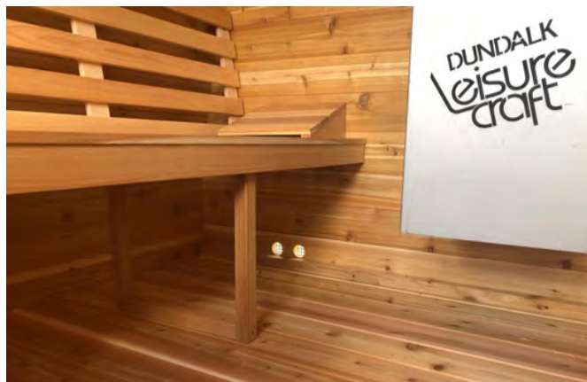
Inlet beside wood heater on Back wall
