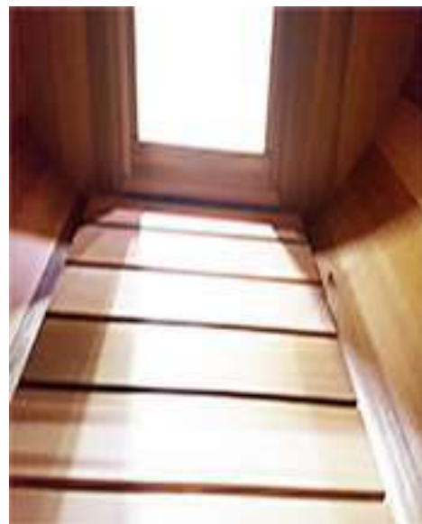
Ensure the flat floor is centered in sauna and that it is level, you can use the door frame to confirm it is level.
