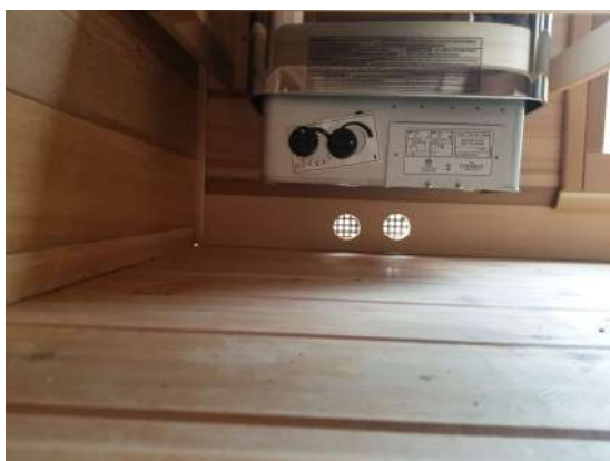
Inlet under electric heater on Back wall
