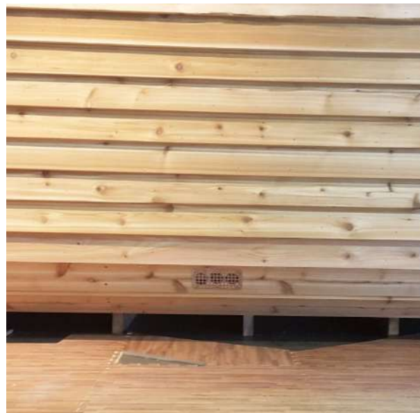
Inlet Vent on side wall under heater (outside)
