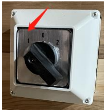
Power to stove heater
