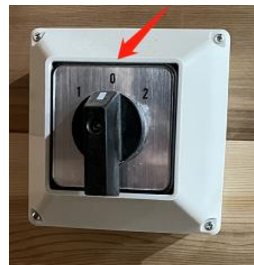
Power turned OFF
