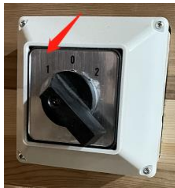
Power to stove heater
