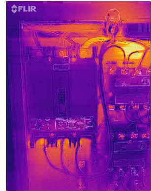
Identify electrical faults
