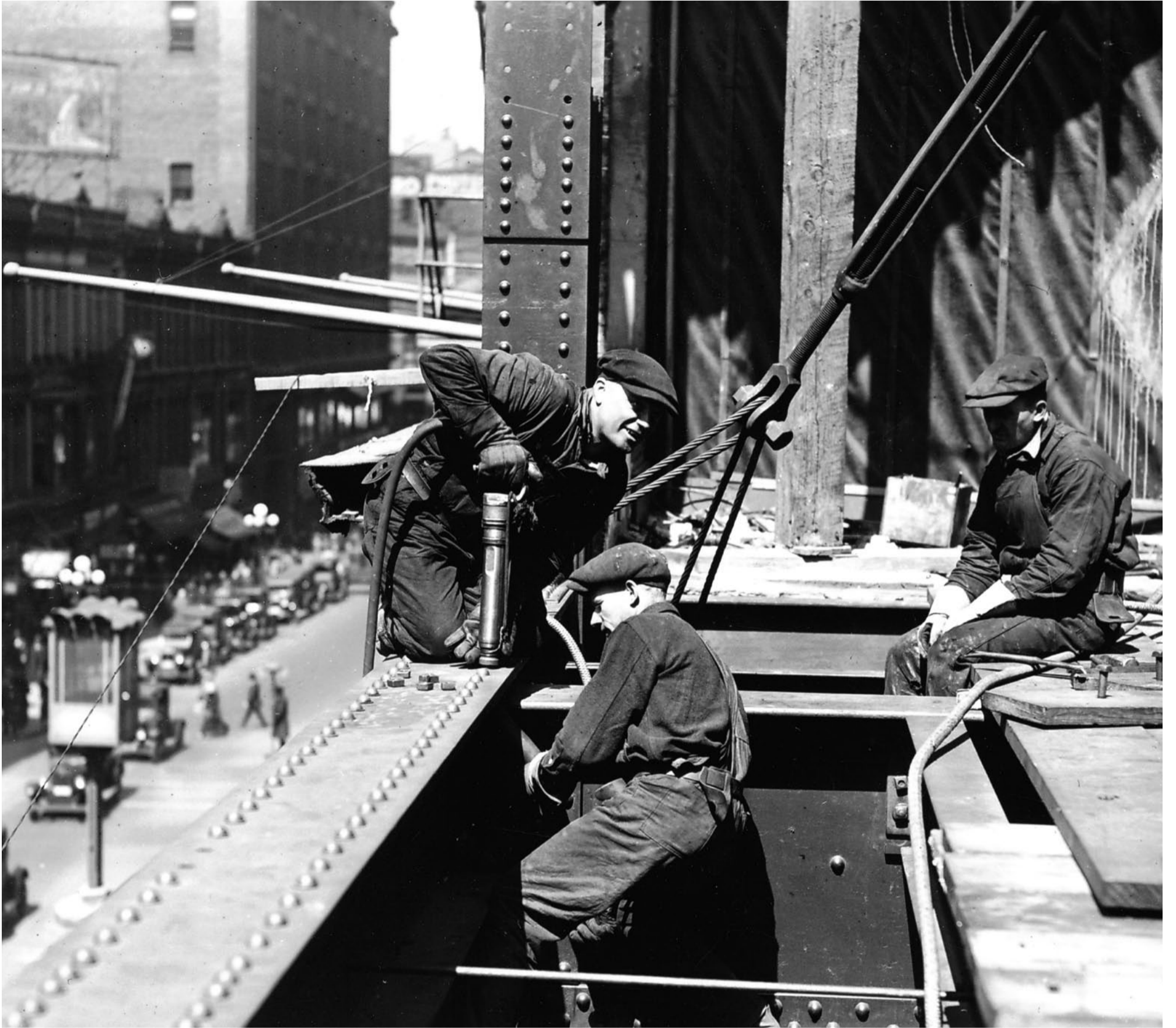
Iron workers at Dayton's building – Minneapolis, Minnesota, USA 1925 Minnesota Historical Society, Photo no.57882 via Red Wing
