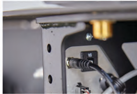
WALL PLUG / CHARGING
