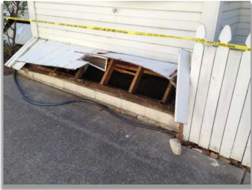
Cripple wall collapsed
