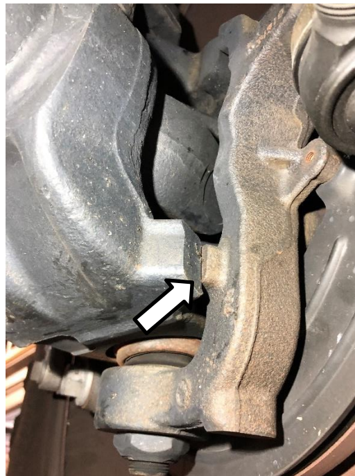
Figure 5. Driver Side Knuckle Fully Turned to the Passenger Side, Contacting the Steering Stop
