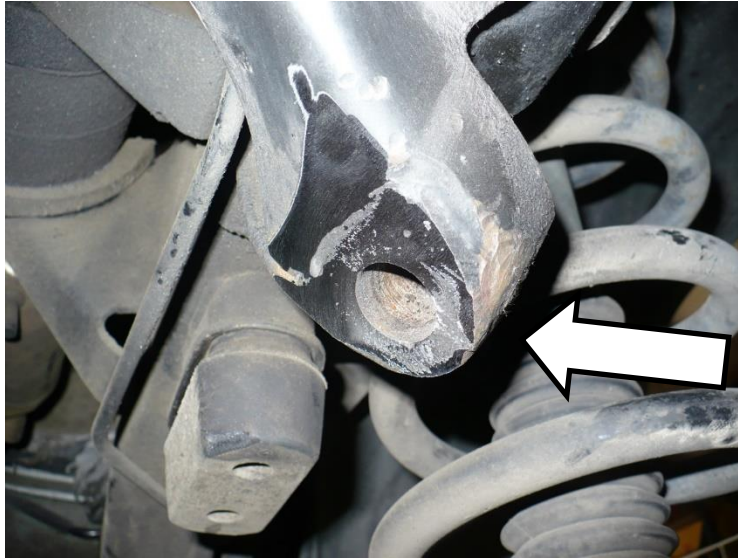
Figure 5. Correctly Modified Underside of Track Bar Mount
