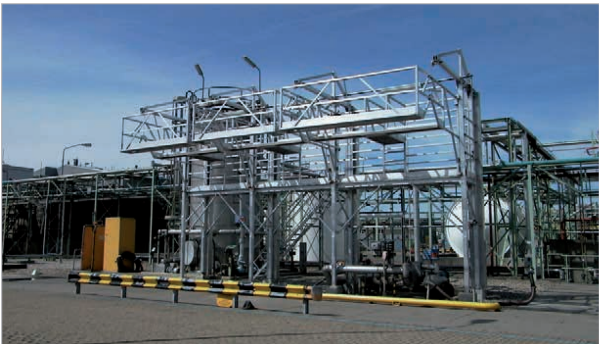
Permanent fall protection loading dock for tankers/trucks
