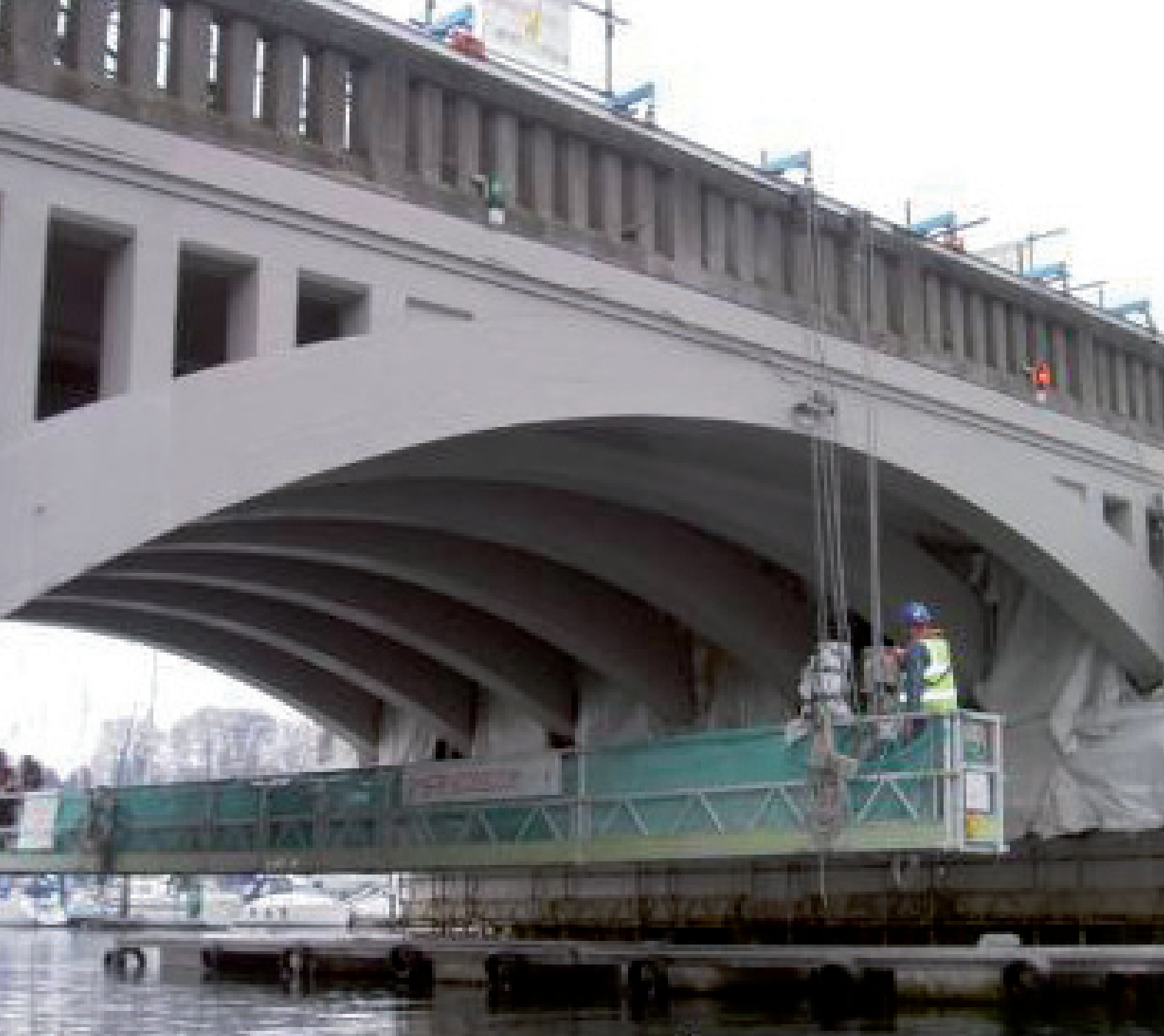
Maintenance suspended platform
