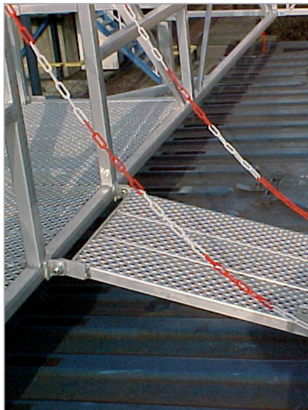
Fall protection system with access to truck roof
