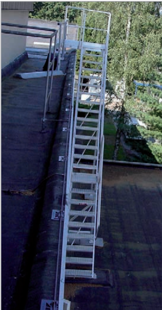
Straight ladder with rest platform and industrial step-over guardrail
