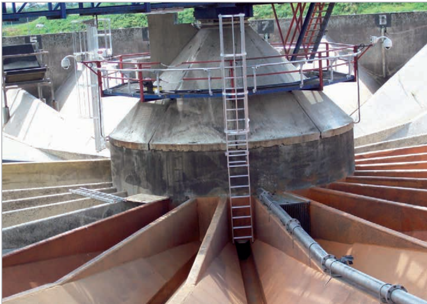
Hoop ladders on rail with step-off platform
