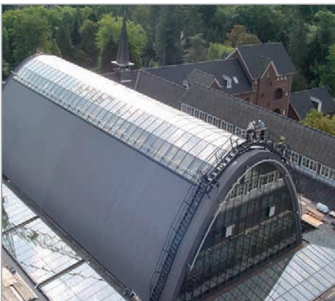
Façade maintenance installation on dome
