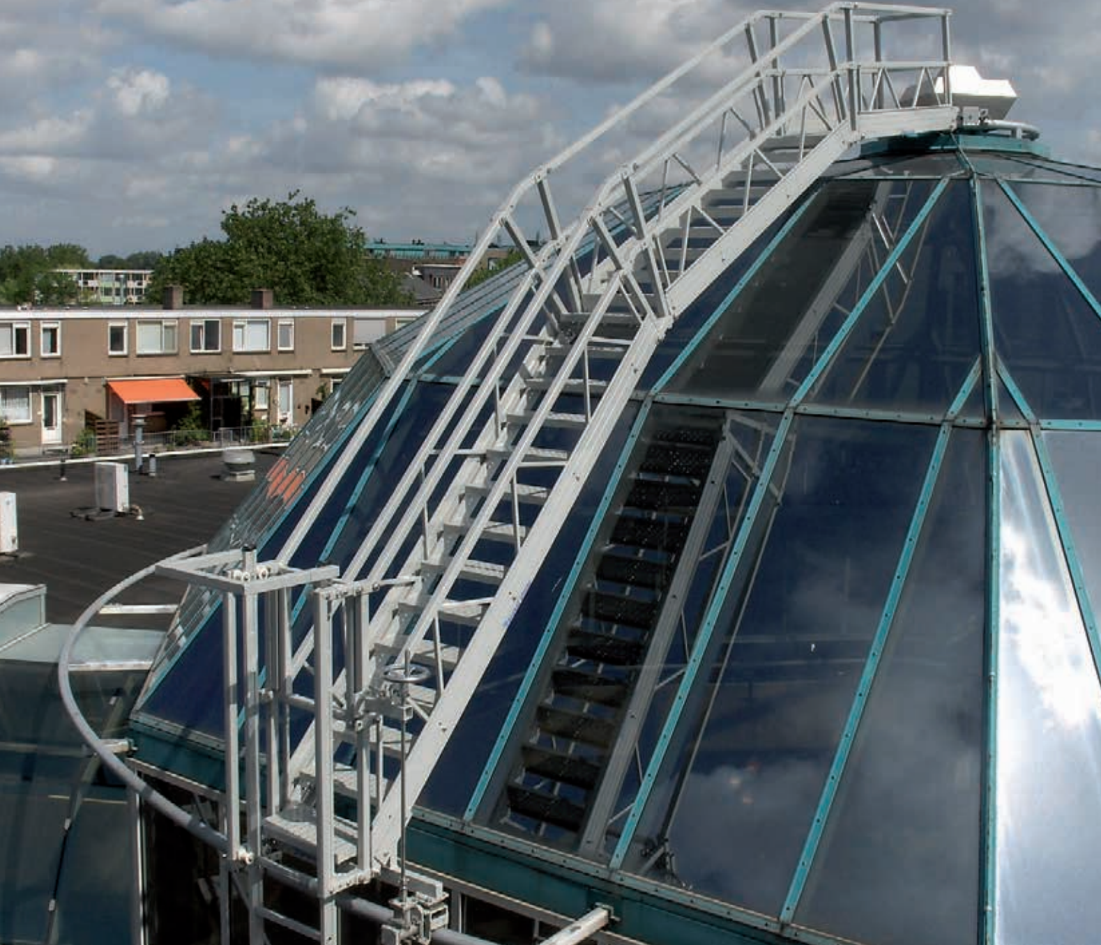
Mobile maintenance platform on glass roof
