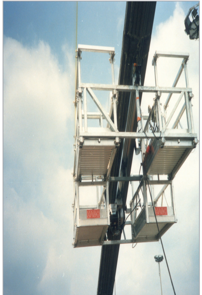
Mobile working platform in a bridge
