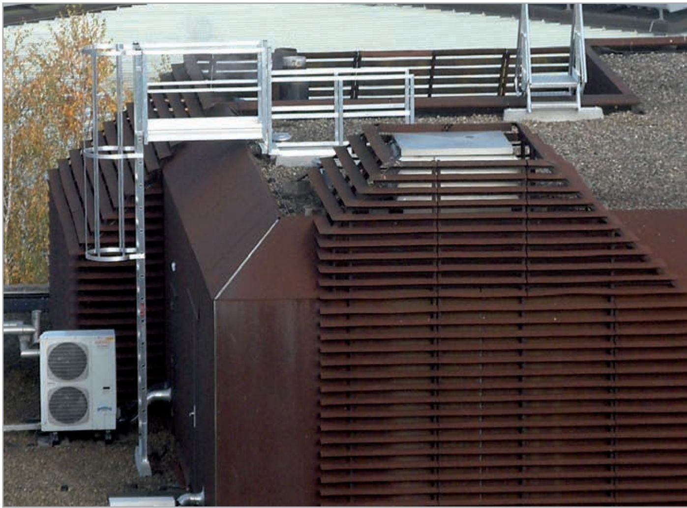
Hoop ladder with industrial step-over guardrail and step-off protection set
