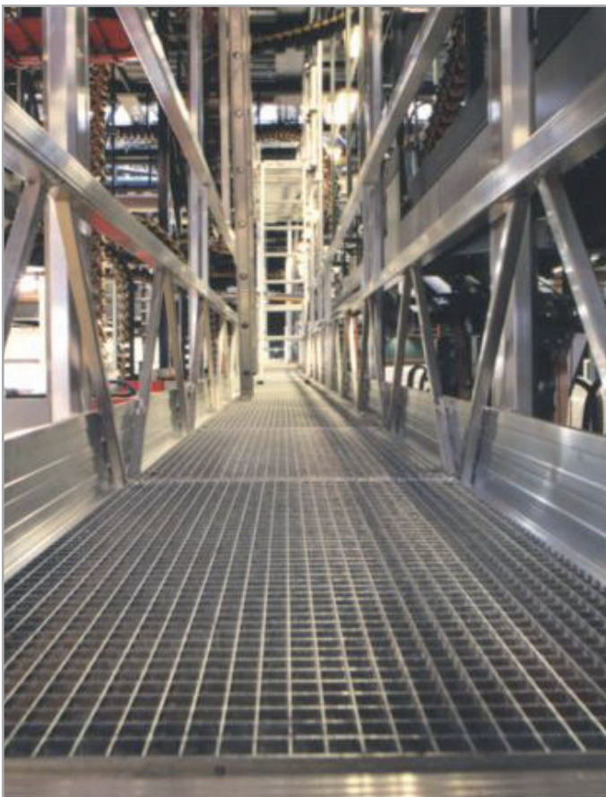
Platform between machines
