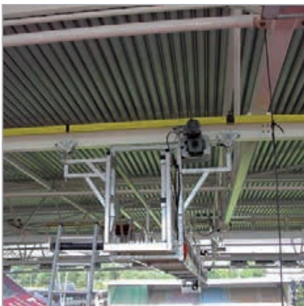
Access door maintenance platform football stadium
