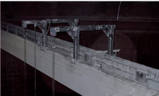
Support arms working platform in silo
