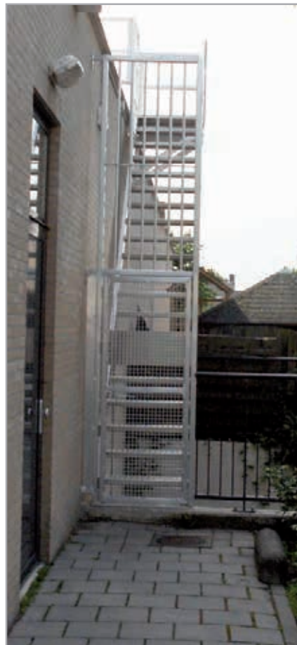
Escape route/fire escape stairs with perforated steps and anti-theft protection railing (with door)
