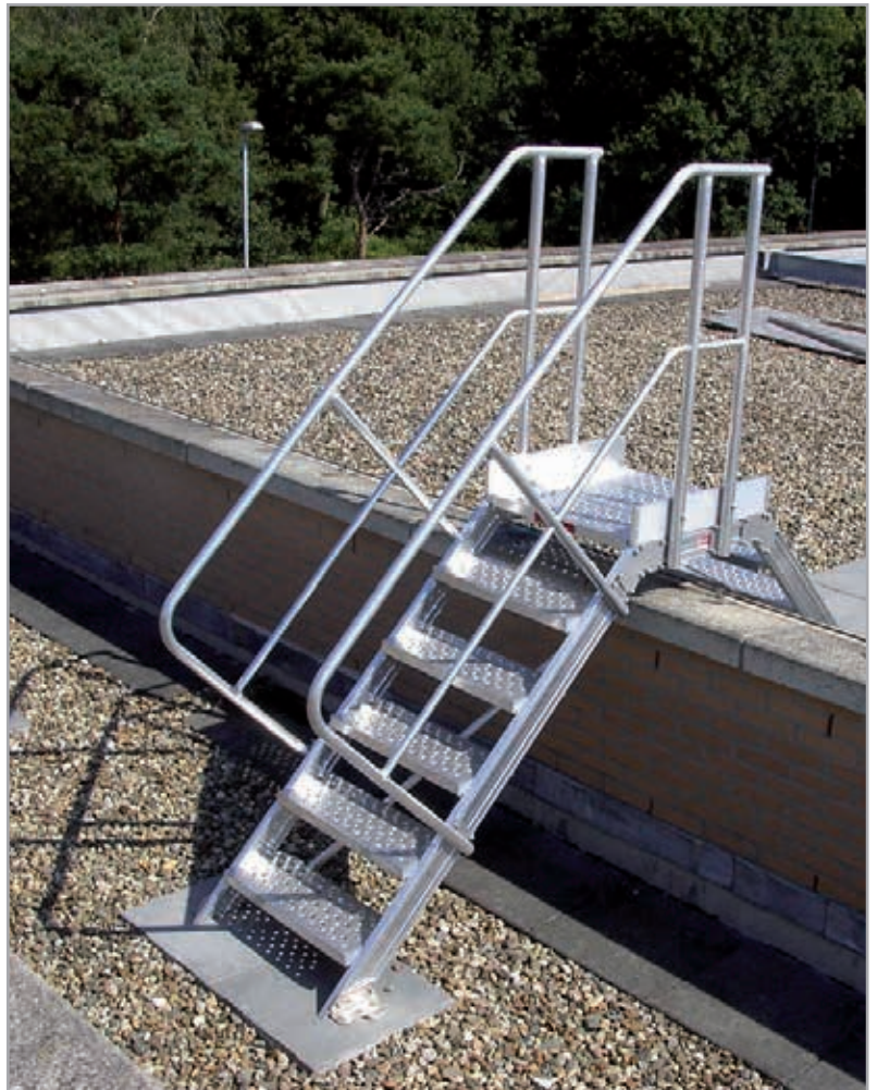
Parapet step-over guardrail
