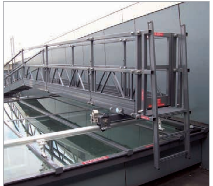
Mobile maintenance platform on glass roof
