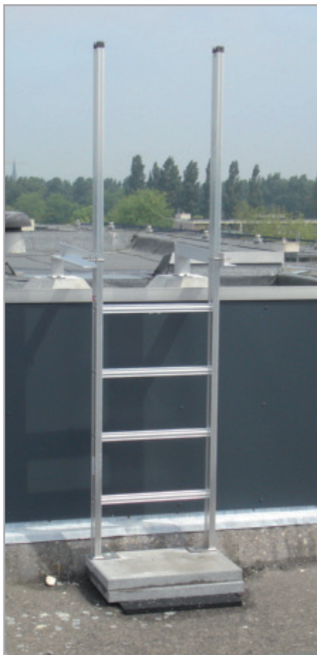
Escape ladder supported separately
