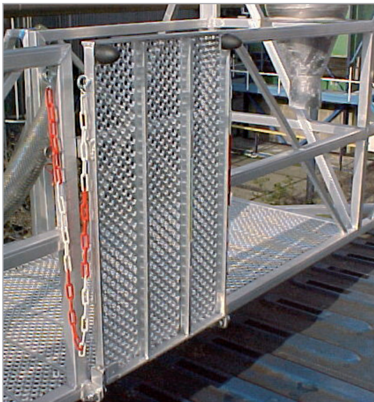
Fall protection system with access to truck roof
