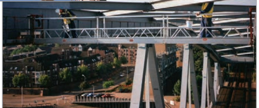
Suspended platform under bridge, with sideways movement (at the bridge over the river Waal in Nijmegen)
