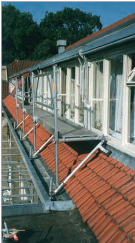
Dormer window scaffold
