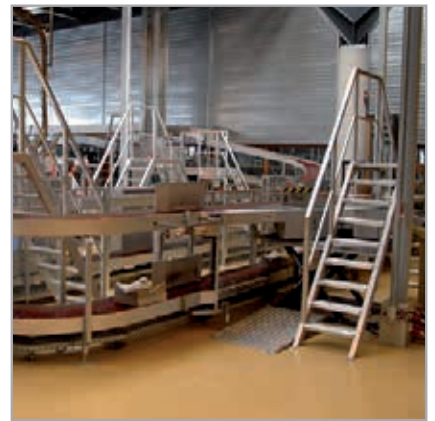
Industrial step-over/stairs for conveyor belt
