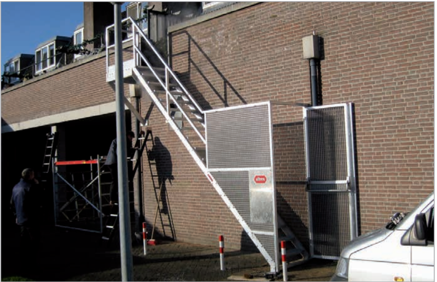
Straight ladder/fire escape stairs with platform and anti-theft protection railing (with emergency door)
