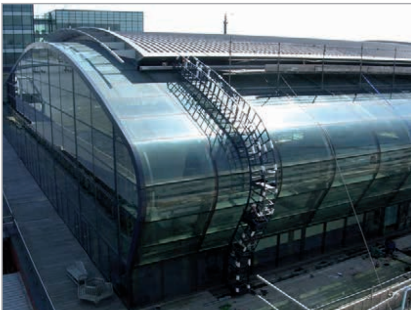
(Semi)circular working platform for façade maintenance
