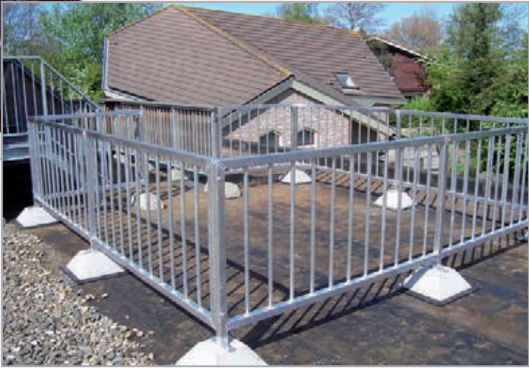
Railing as permanent edge protection
