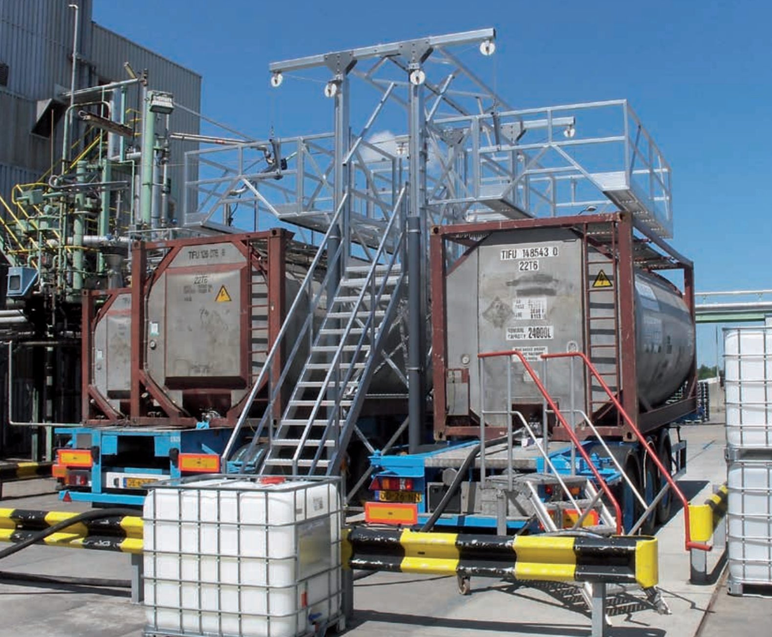
Safety guardrail system for tankers (during loading)
