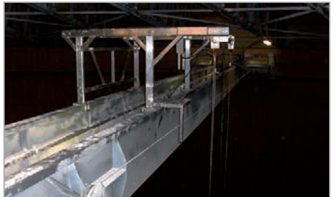
Support arms working platform in silo
