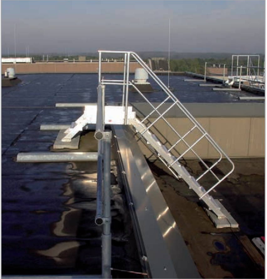
Straight ladder with parapet step-over guardrail
