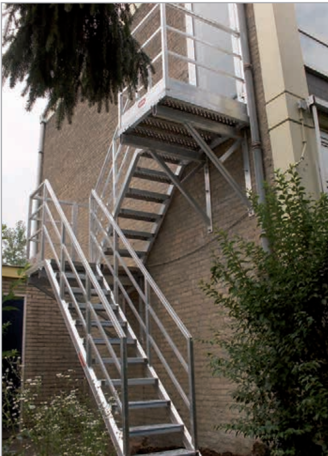
Fire escape stairs with rest platform for use as an escape route
