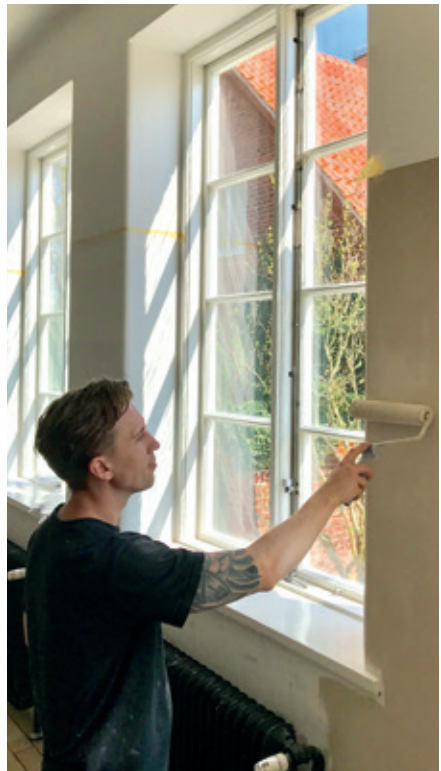
Fill and paint with Linus Wall Paint. Use a yarn roller or brush. Use a wide spackle knife or roller with Linus filler for skim coating (see page 19).
