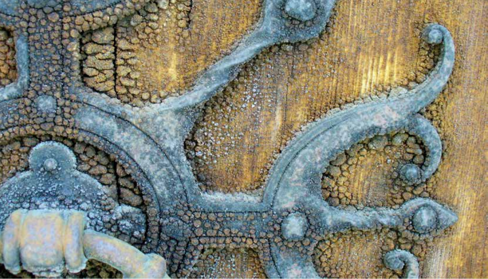
maintenance of tjärskiktet long time builds a characteristic pattern, when the substrate is saturated and tar moves with temperature. Photo: Arja Källbom.
