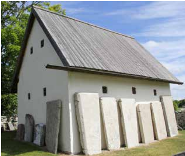
South of roof on Fole parish magazine. Photo: Arja Källbom. Testtak at
