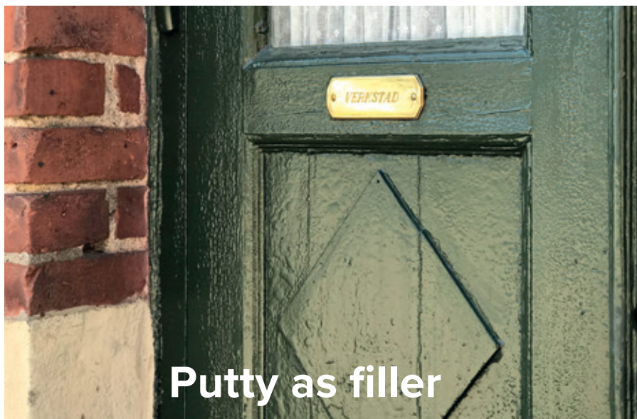
Door from 1926. Easy "anti-aging" measure for 100 years. Linseed Oil Putty in cracks. Painting an old surface with new Linseed Oil Paint.
