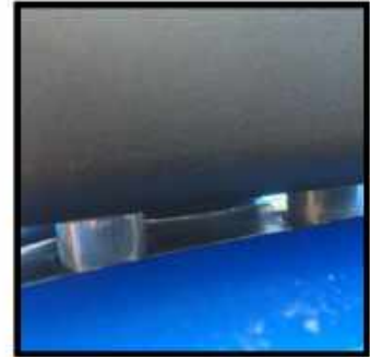
After installing the spacers with silicone as shown in the steps on the previous page re-install the weatherstripping
