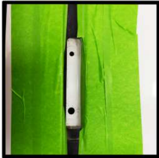
View of bottom hole drilled, be sure to clean any shavings away that fell thru while drilling.
